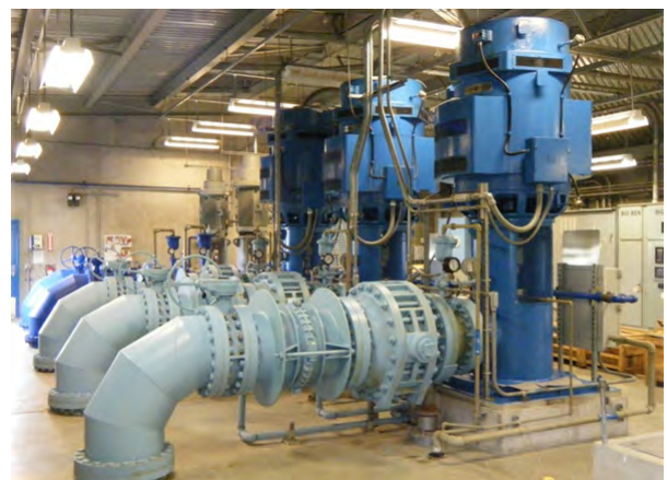
Finished water pump station at JWC WTP
