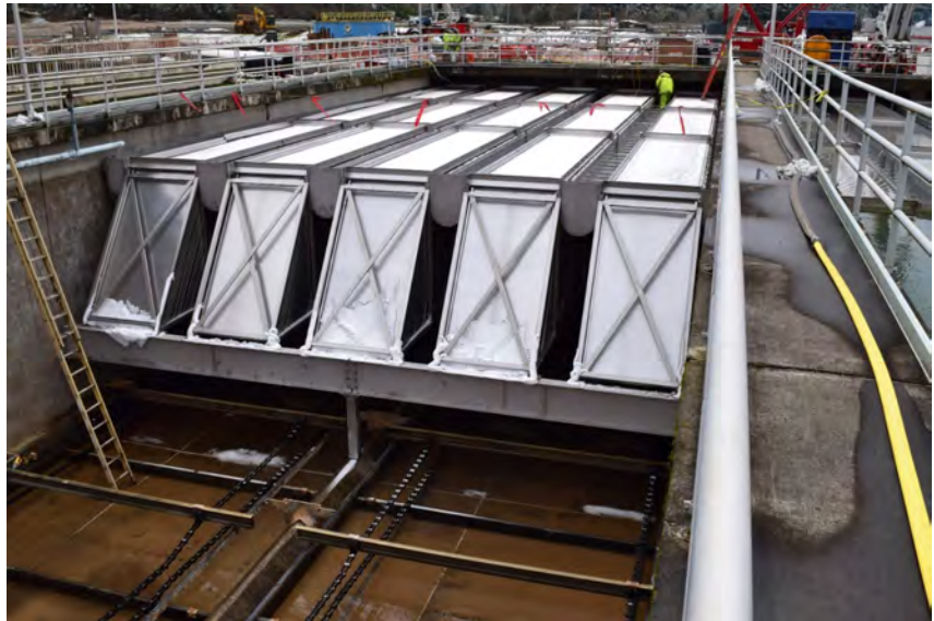
Plate settlers installed at sedimentation basins
