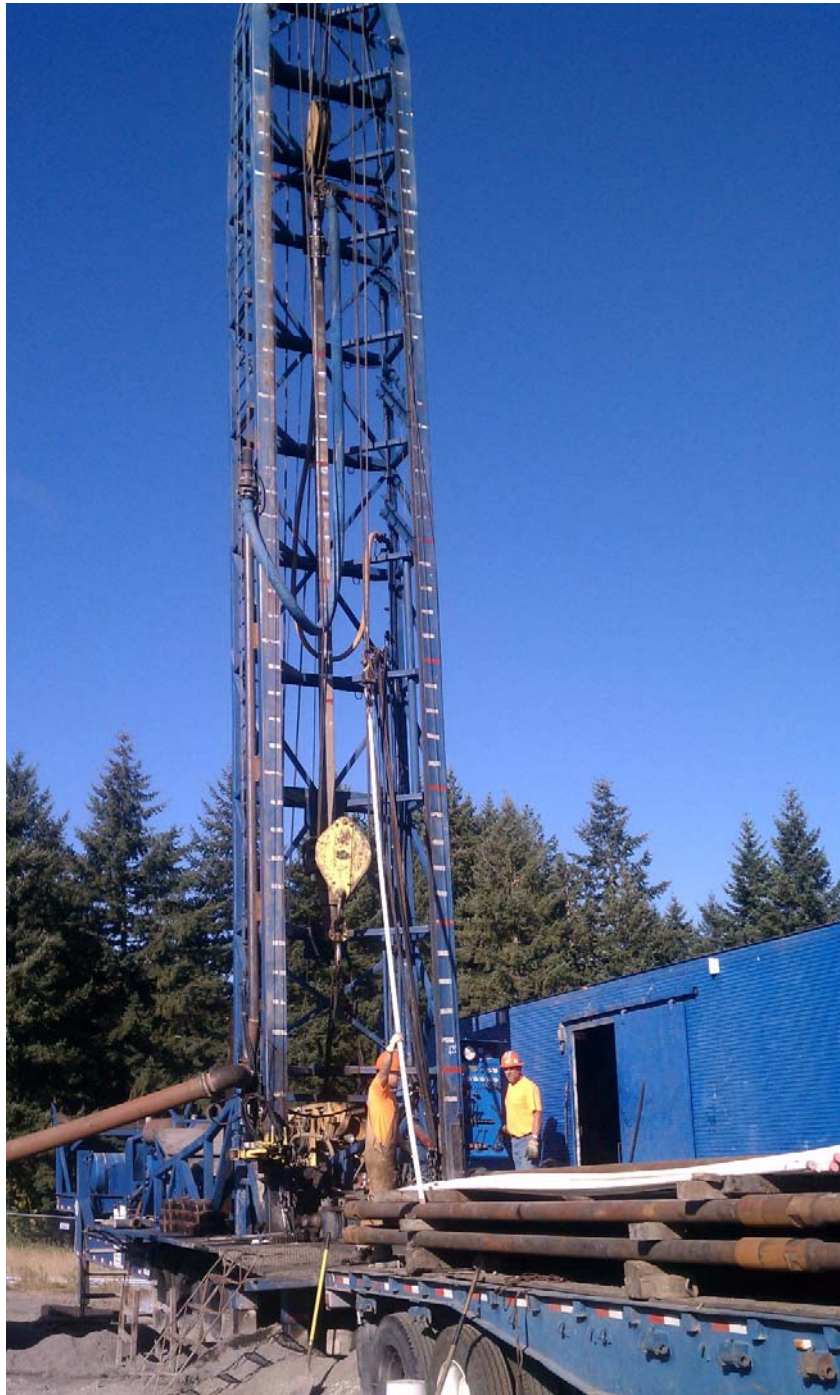
Drill rig used during Aquifer Storage and Recovery (ASR) Feasibility Study in Spring 2011.
