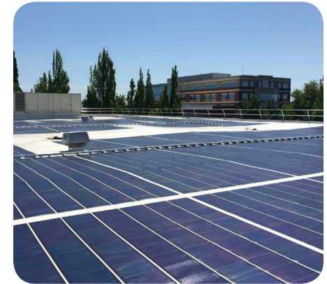
This 65 kW thin film solar array is installed on the roof of the Washington County Public Services Building.
