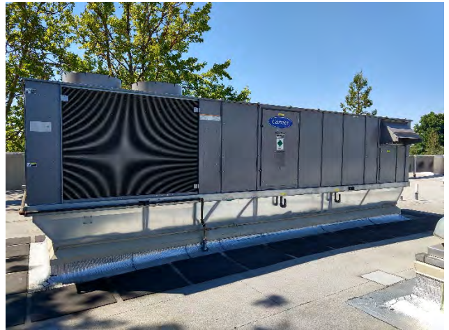
Air Handler on Juvenile Services Building
