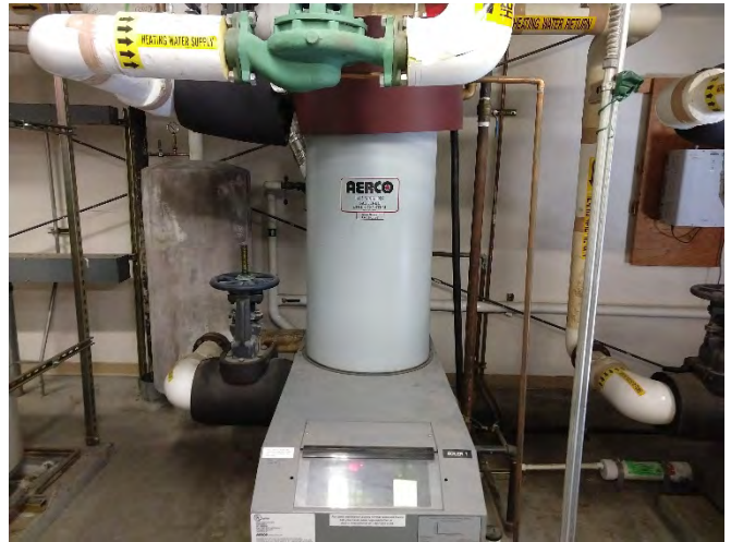
Hot water heater in the Justice Services Building
