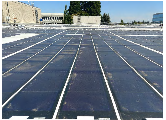
Solar Array on roof of Public Services Building
