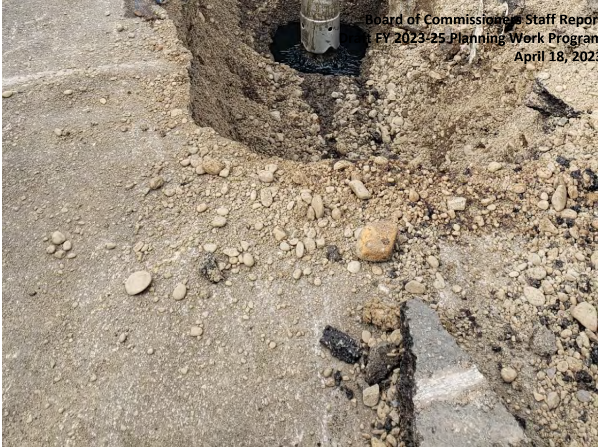
Removing gasoline that spilled from an underground storage tank at Highway 99 and Main Street in Monmouth in April 2021. [Department of Environmental Quality]
