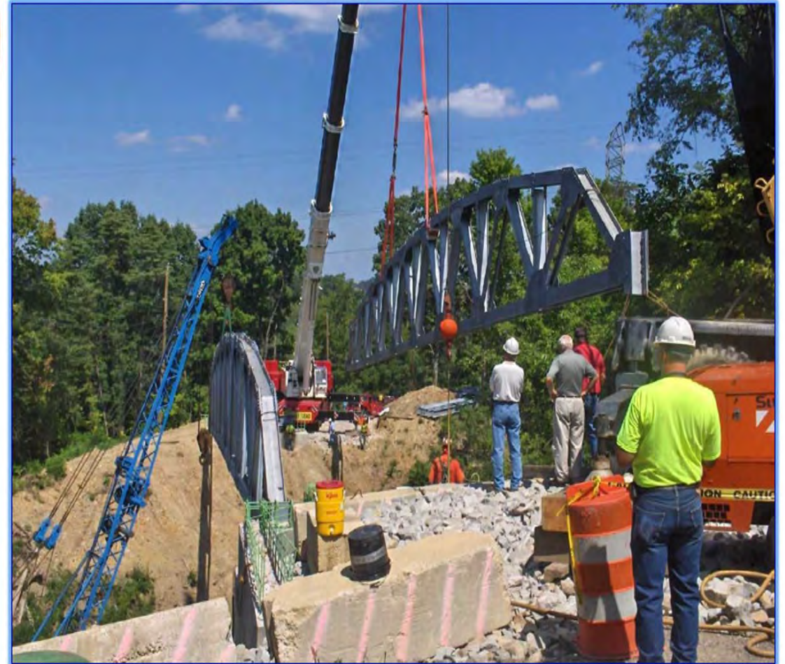
With first truss secured, the second truss is ready to be set.
