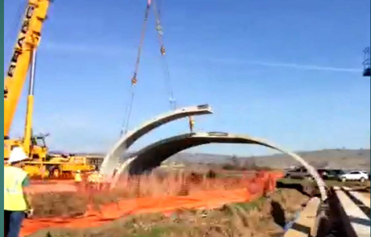
Rotate Arch Units are set on foundation and matched with companion arch
