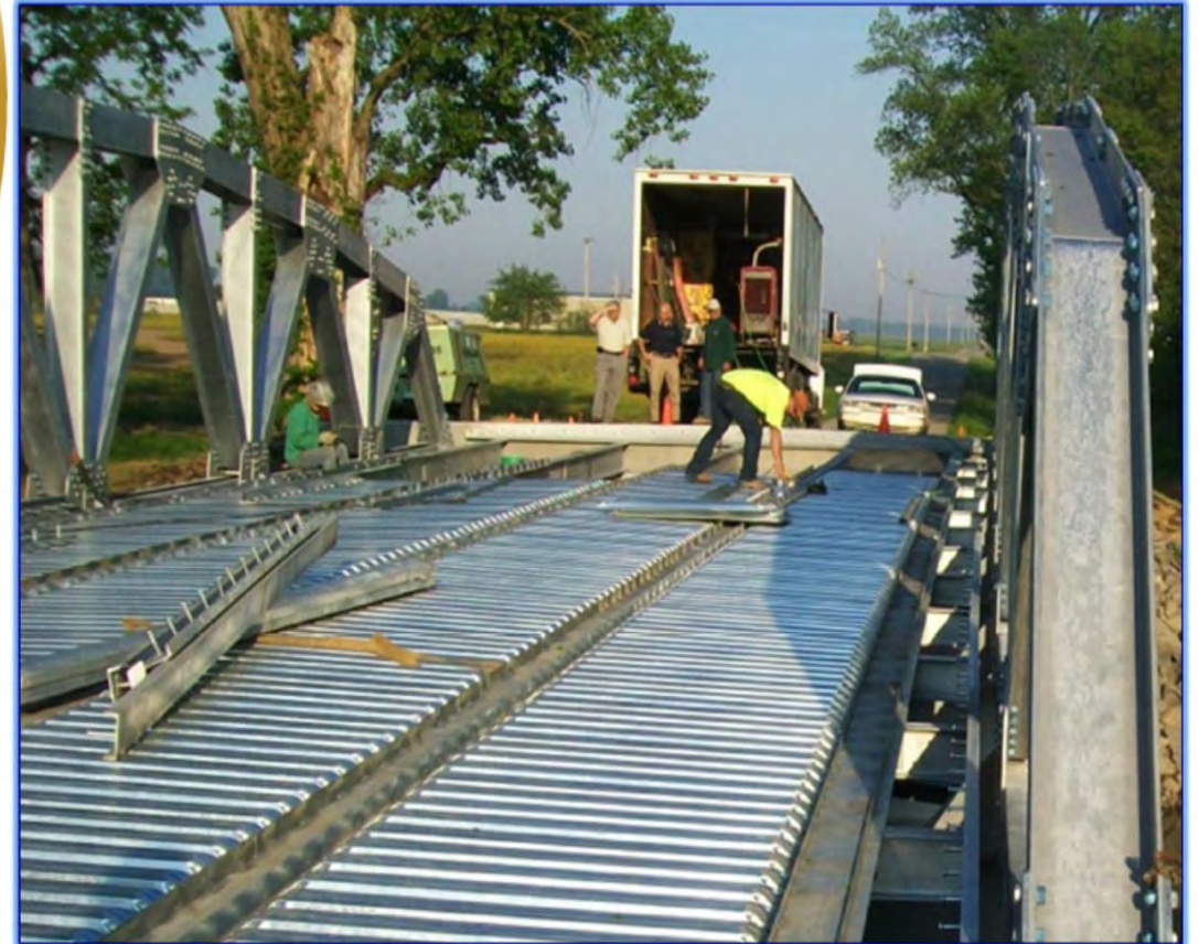
After all structural steel is installed and tightened to specification the deck is placed. Here we see SIP forms for concrete deck.
