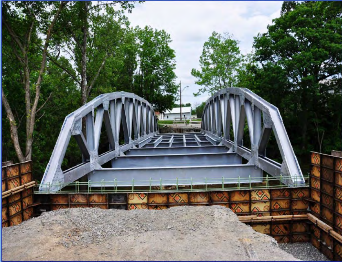
After all floorbeams have been installed and bolts tightened, stringers are placed.
