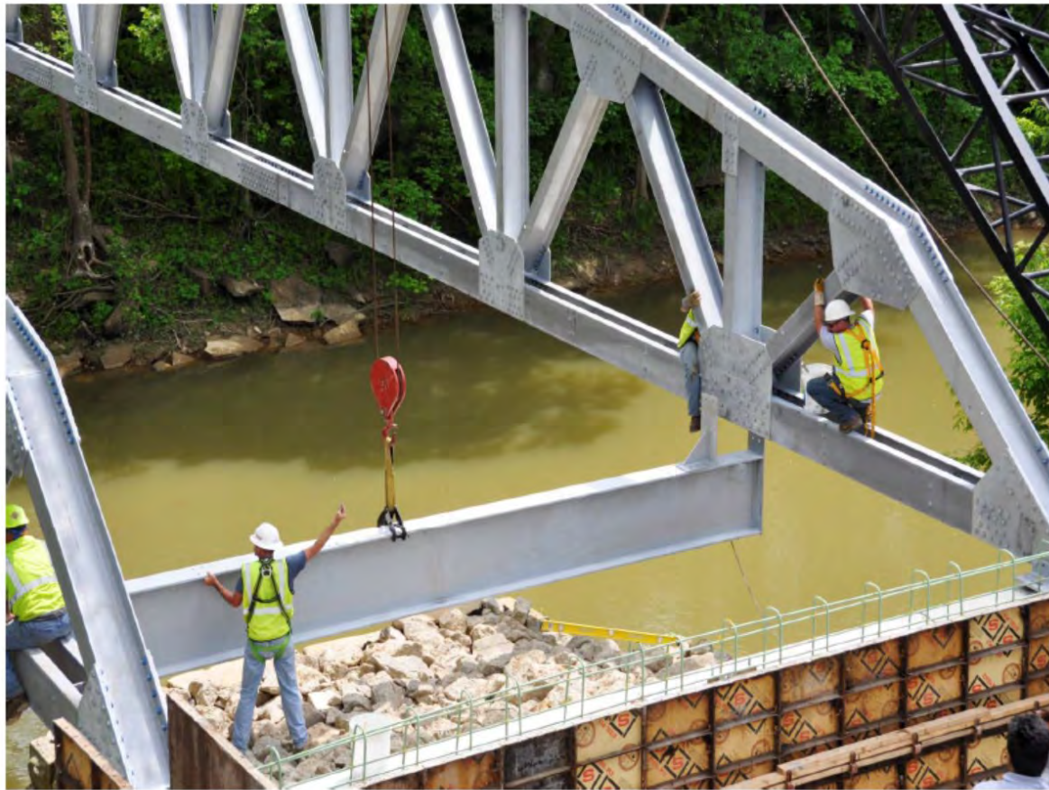
With both trusses set and secured onto bearings the first floorbeam is set
